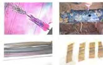
Fig. 1. Different examples of power cables insulation degradation. The insulation defects may occur from poor installation from the beginning on or may be initiated during the service life of a cable system.
